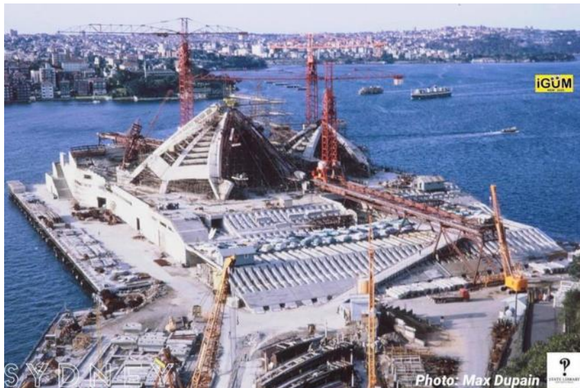
60 years ago, on September 2 nd 1964, Sydney Opera House construction progress pictured from 'Unilever House' rooftop.
